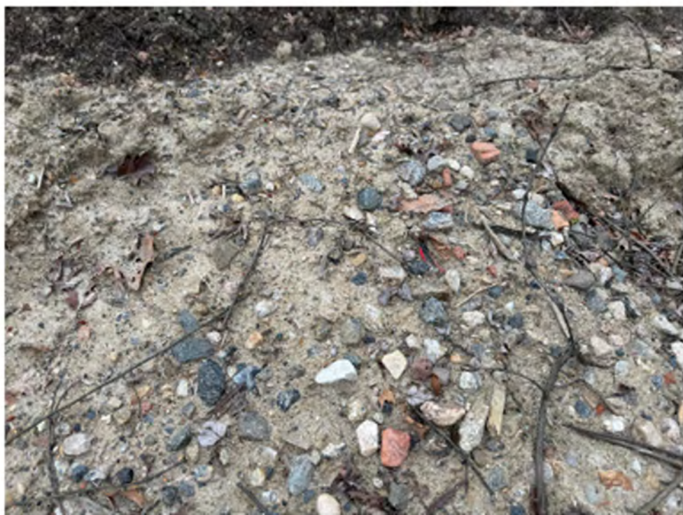
Photo 9: View of fines and rocks present on the surface of the berm material.
